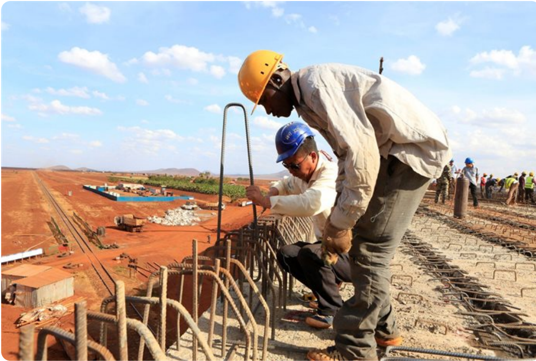
A Chinese engineer and a local construction worker work on a section of the Mombasa-Nairobi standard gauge railway (SGR) in Eruli, Kenya. Reuters/Noor Khamis
