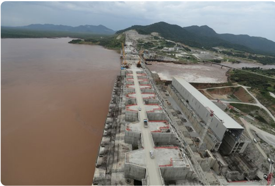
Ethiopia's Grand Renaissance Dam is seen as it undergoes construction work on the river Nile in Guba Woreda, Benishangul Gumuz Region, Ethiopia, 26 September 2019. Reuters/Tiksa Negeri
