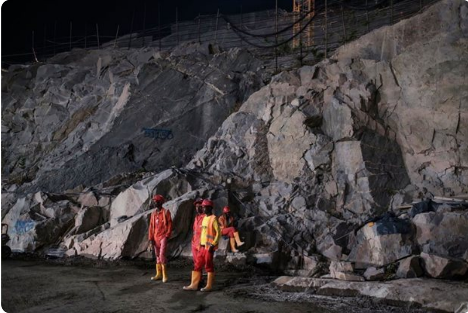
Construction workers stand next to rock wall at the Grand Ethiopian Renaissance Dam in Ethiopia on December 26, 2019.
