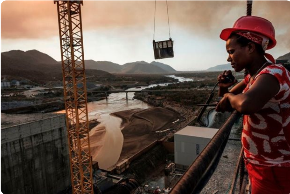
The Grand Ethiopian Renaissance Dam, a 145-metre-high, 1.8-kilometre-long concrete colossus is set to become the largest hydropower plant in Africa. (Photo by Eduardo Softeras/AFP via Getty Images)
