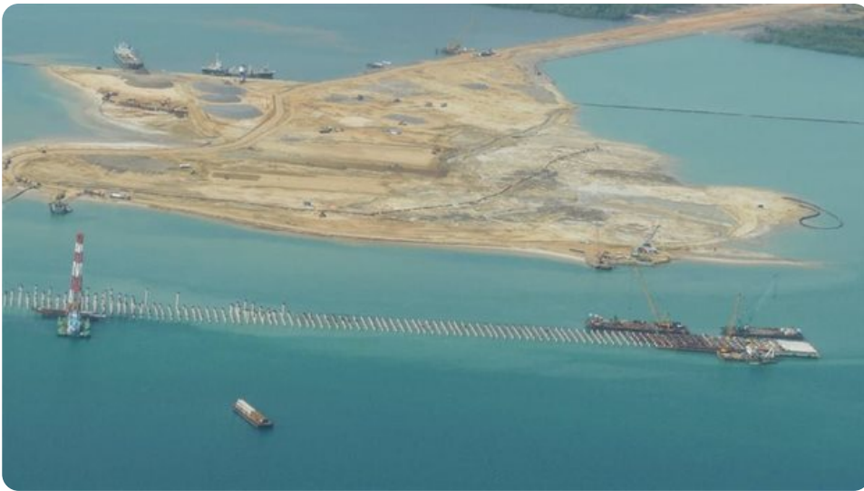
Construction underway of a new port at Lamu, Kenya. Michael Edward Walsh/flickr , CC BY-NC-ND
